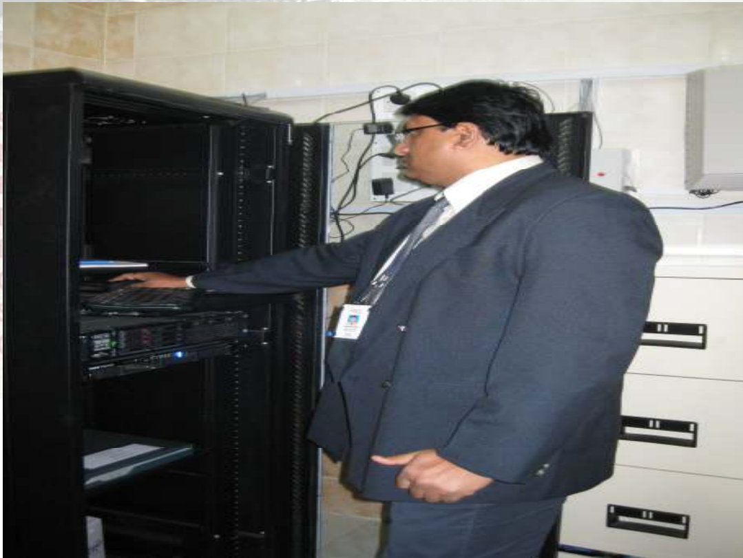
Picture 4: Mr. Koushik Ghosh of Axsys working at MSCL Server Room for FMS Deployment
